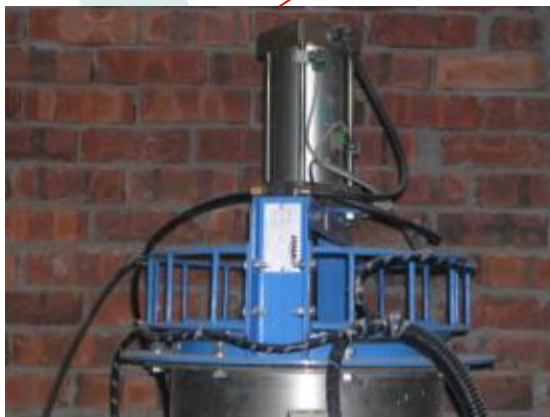
Primary Air Intake
