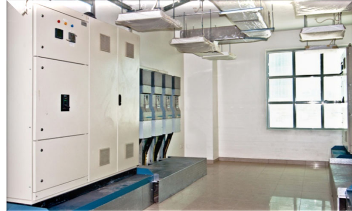
Main Control Centre
