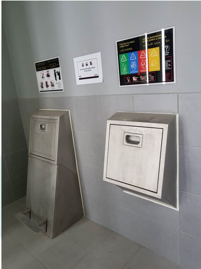
Gravity Vacuum Load Station on every floor of residential units
