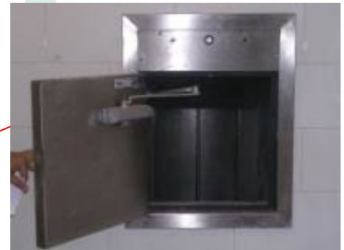
Load Station Door
