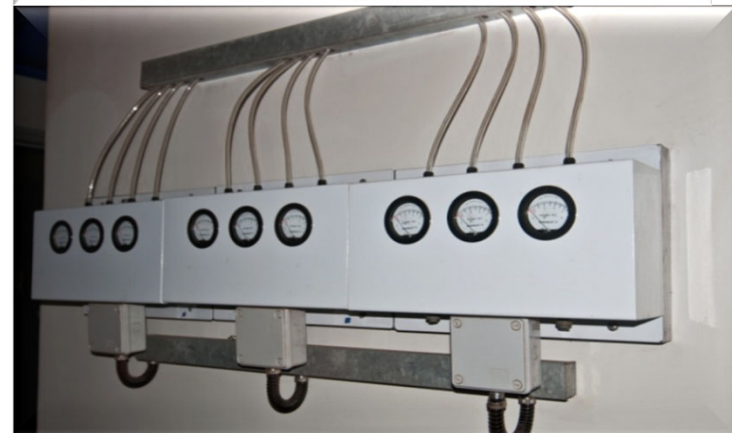
Pressure Differential Gauges
