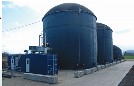
Aerobic Digestion Plant
